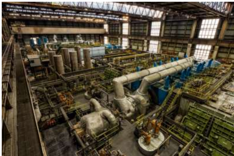
Rugeley Power Station's turbine hall (from the company's digital material, now in the service's collections).
